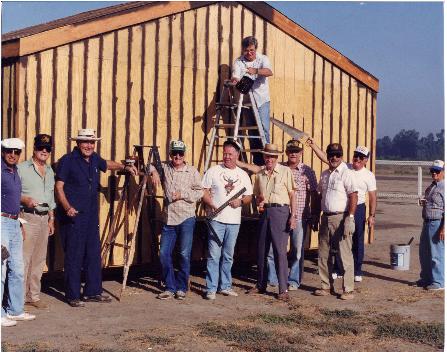
Photo of the completion of the Club House, early 1991. Chuck Colwell was in the photo and he left the area in the spring of 1991.
